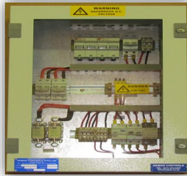
Figure 4: Solar System Distribution Board with circuit breakers
