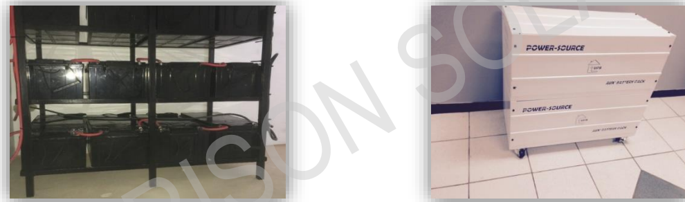
Figure 3: Battery bank with battery rack
